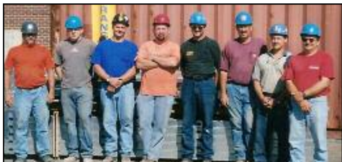
Biter Electric crew at Penn State Health and Wellness Building. L to R: Jack Horner, Pat Kopera, Tyler Slegel, John Lynch, Howie Wright, Russ Aumiller, Steve Umstead and Jeff Biter.
